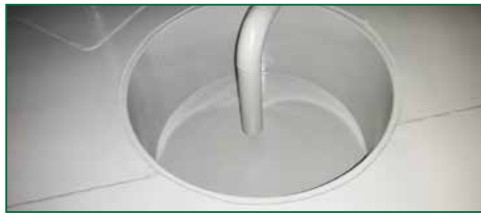
Novocoat SP2000AR Ceramic Coating lining in a tank sump
